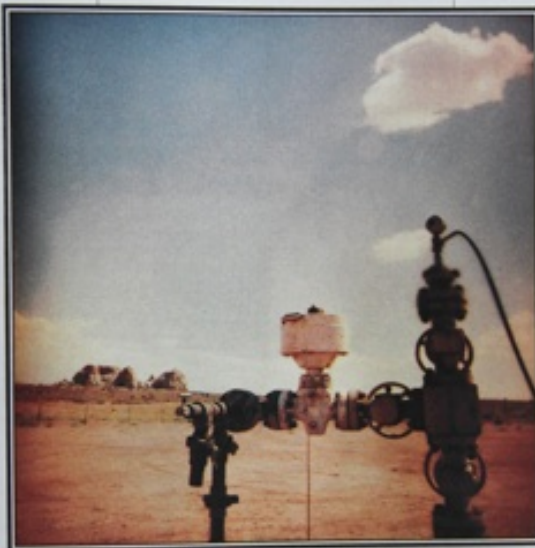
Oil well located on federal land for which SUWA seeks wilderness designation
